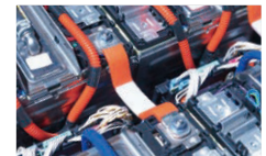
Connection resistance of battery busbars
